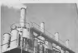
BUILT IN 1935, these precipitators prevent acid from entering the atmosphere. Electrodes carrying 75,000 volts separate acid which runs down stacks to be reclaimed.
